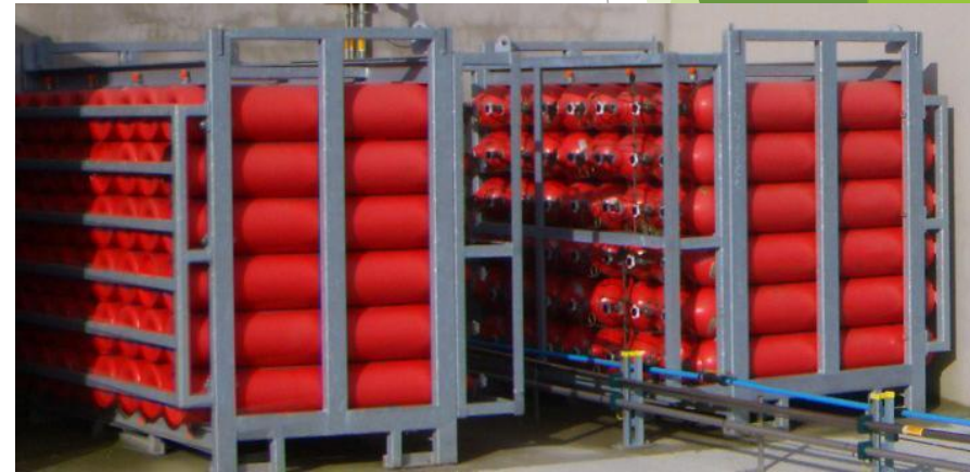
Hydrogen in gaseous form storage tanks
