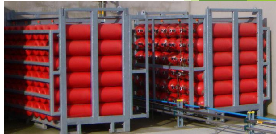
Hydrogen in gaseous form storage tanks
